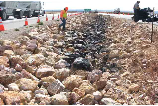
Oil and Diesel Spill Treatment
